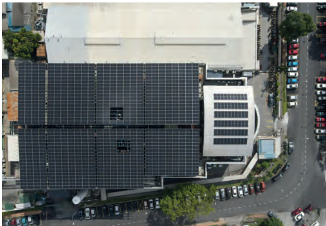
Figure 21: Rooftop solar panel system
